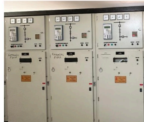
Figure 28 Circuit Breaker Room
