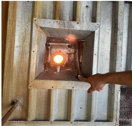
Figure 11 Burning fuel inside the boiler
