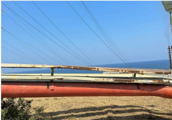
Figure 1 Fuel transportation pipes
