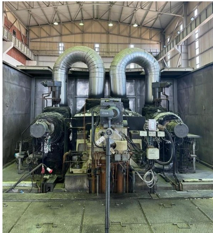
Figure 12 Generator Part of the Turbine
