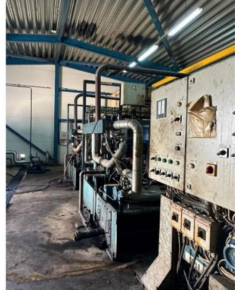
Figure 24 Fuel Separator Room
