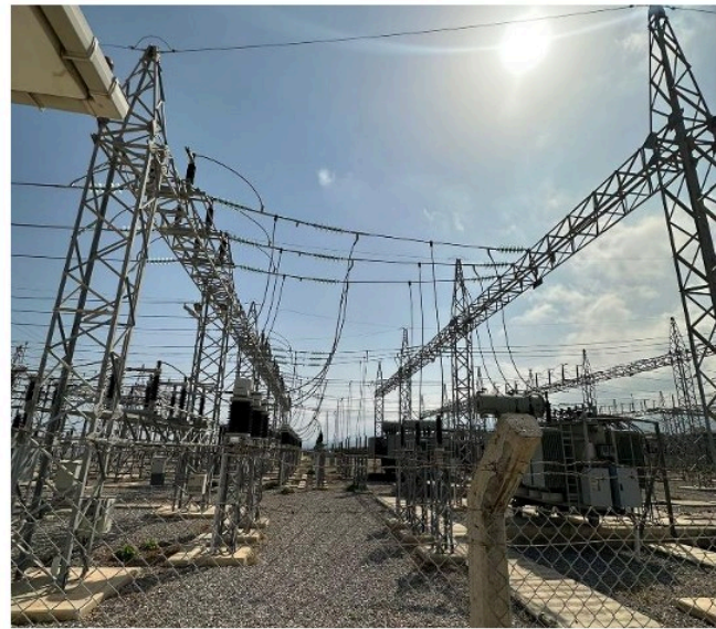
Figure 40 Step up Transformers to transport electricity easily
