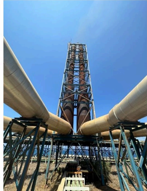
Figure 22 Exhaust gas going through the chimney
