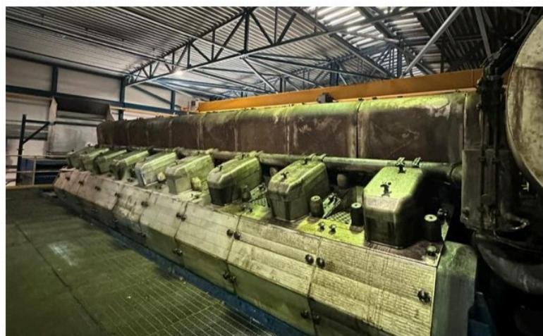
Figure 21 Diesel Generator Piston view in different location
