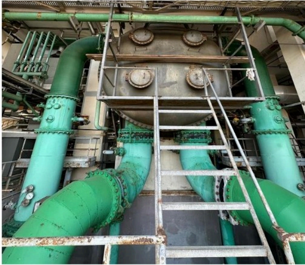
Figure 14 Condenser view from front
