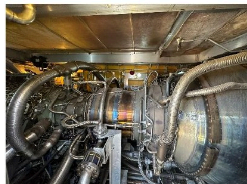
Figure 30 Gas Turbines inner view
