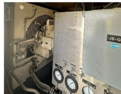
Figure 31 Gas Turbines Pressure Room
