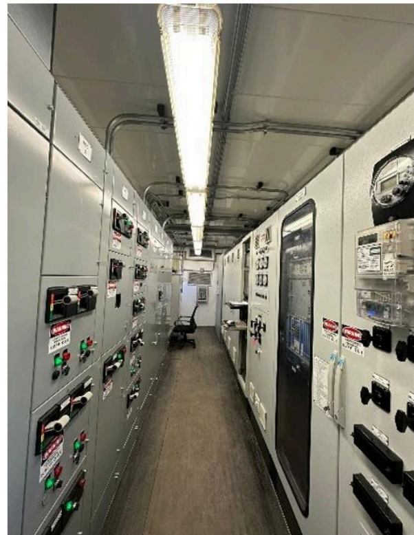
Figure 33 Control Room of Gas Turbines
